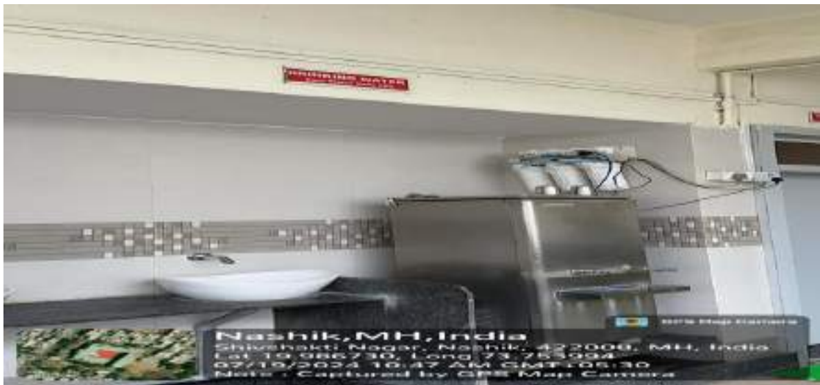
Drinking Water Facility
